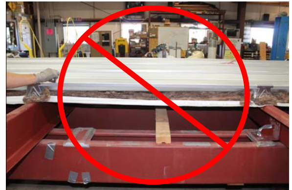
Improper Insulation at Mid Span (Fig.4)
